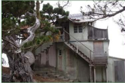
"Before" showing the deteriorated condition.
