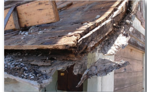
Much of the roof decking had rotted away (Without applying the normal layer of waterproof roofing paper, Pedro had nailed chicken wire directly to the roof decking)
